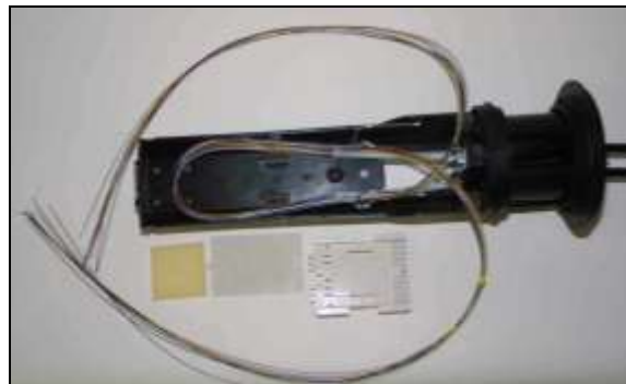
Figure 7 – 2600LG closure with slack fiber stored in the fiber storage area.
