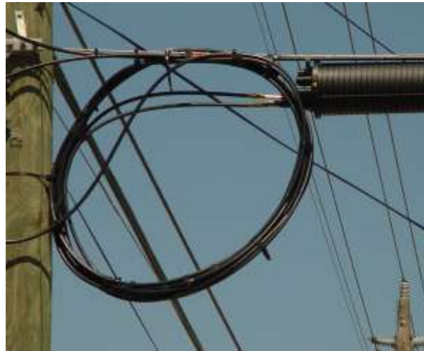
Figure 4 – Slack Storage Coil
